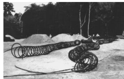
Svec collectors for a school in the Toronto area; the spirals are made ready for installation in the trenches.
