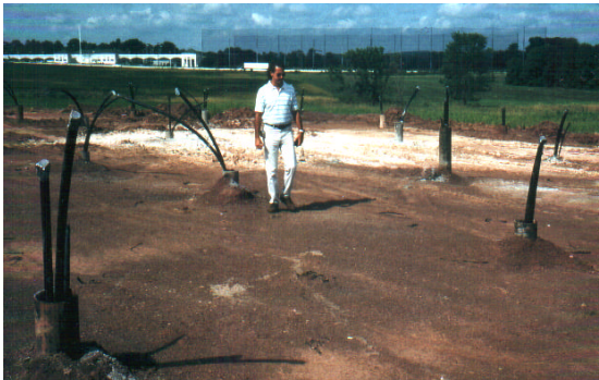
Borehole heat exchangers („wellfield“) for a school in Northern New Jersey, USA
